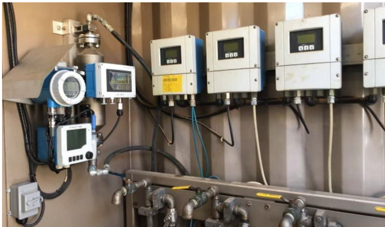
Promass I 300 flow valve installation in a Gore Nitrogen quality control unit
